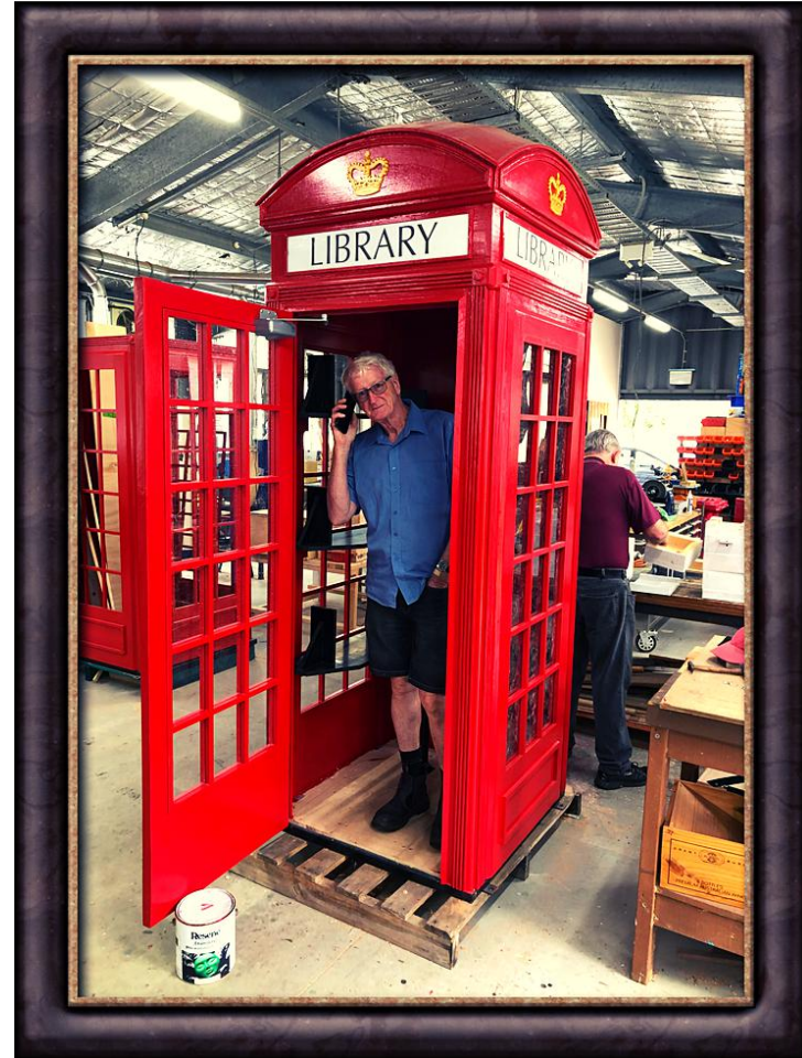
Peter Hall one of the tradesmen who helped built the Red Box ironically takes a personal mobile whilst completing work on the first of the two Red Boxes.
